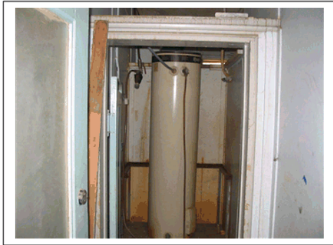
Plate 19 : Fibre glass insulation to Hot Water Heater of the Offices Areas (West) – Cannery Building
