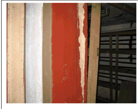
Plate 15 : C & D Building – architrave to cool room in sprinkler room – poor condition ( Sample Pb1 : 34% - Lead Paint).
