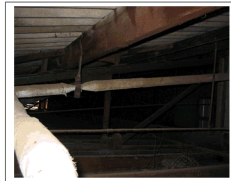
Plate 4 : Pipe Lagging in roof space of the South Offices of the C & D Building
