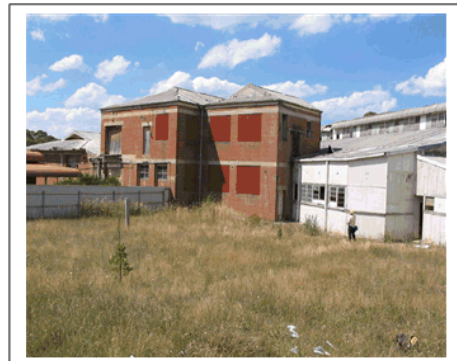
Plate 18 : View of C & D Building to the North – shows low paint use on asbestos cement sheet.
