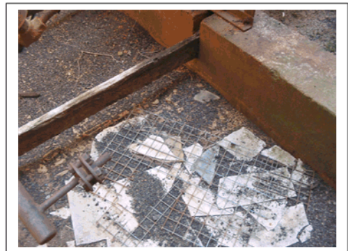
Plate 8: Asbestos Sheet Debris
