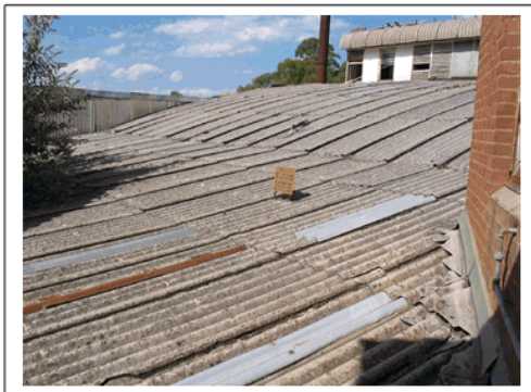
Plate 7: C & D Building: Asbestos Corrugated Roof Sheet from the Loft
