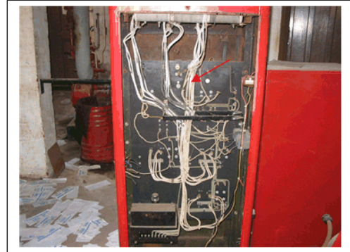
Plate 14: C & D Building – Sprinkler Room – Cable Sheath on cables in control panel of Compressor No. 1
