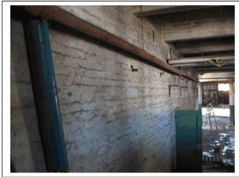
Plate 1 : Pipe lagging to 'Old' Hot water pipe in C & D Building (western side).
