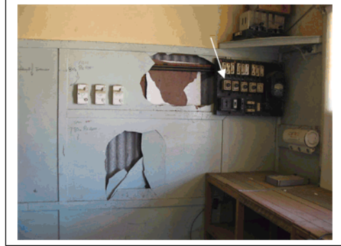
Plate 10: Display Centre – Cracked internal wall sheet and Electrical Switchboard Backing Sheet
