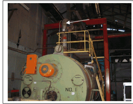
Plate 2 : Pipe Lagging to elbow above Boiler No.1 in Boiler House
