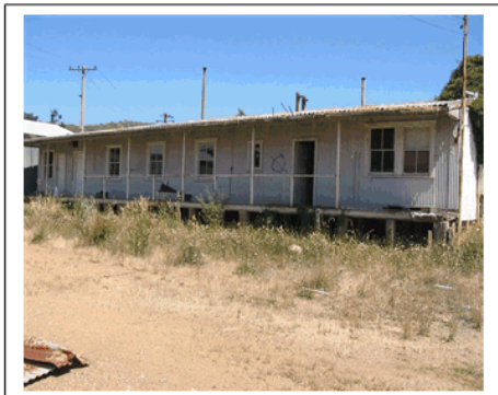
Plate 17 : Display Centre – Verandah Woodwork ( Sample Pb1 : 3.4% - Lead Paint).
