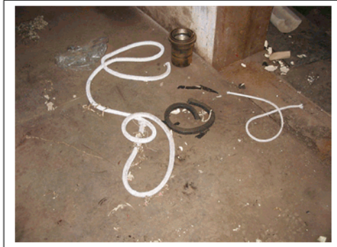
Plate 13: C & D Building – Sprinkler Room – Loose Valve Packing
