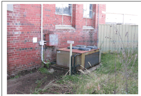
Plate 24: Air Conditioning Unit
