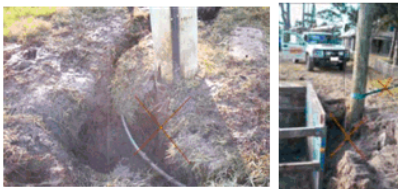
Above: Poles with become unstable if undermined
