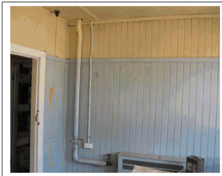
Plate 3 : Pipe Lagging to Hot water pipe in south west office of the C & D Building
