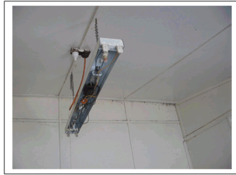
Plate 22 : PCB Capacitor Light Fitting in the Display Centre
