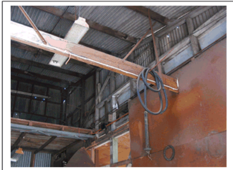
Plate 23 : Assumed PCB Capacitor Light Fitting in C & D Building
