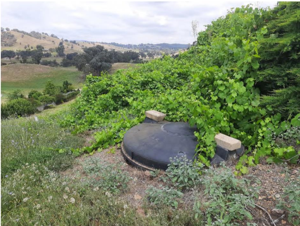
Figure 3 – Polymer septic tank discharging into unmaintained and overgrown absorption trenches (Photo: P McCarthy / Snowy Valleys Council)
