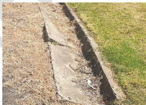
Figure 3-23 Damaged Kerb (Simpson Street)
