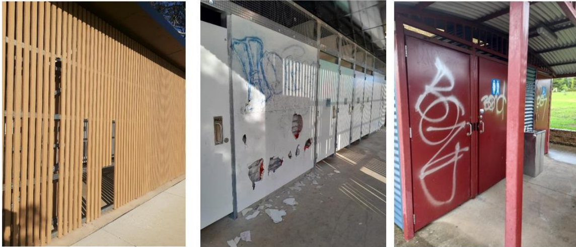
Photos of Pioneer Park and Richmond Street – Tumut Playground - vandalism 5 March 2023
